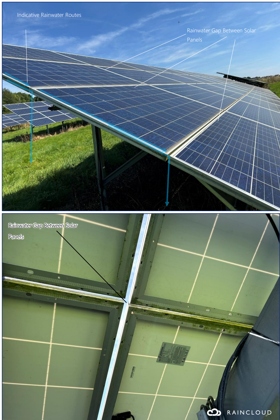
Plate 12-25 Rainwater gaps on PV array table
